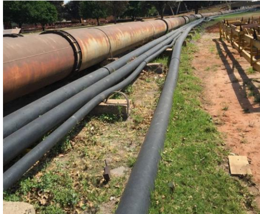
Figure 1: Current pipelines at Power Station
